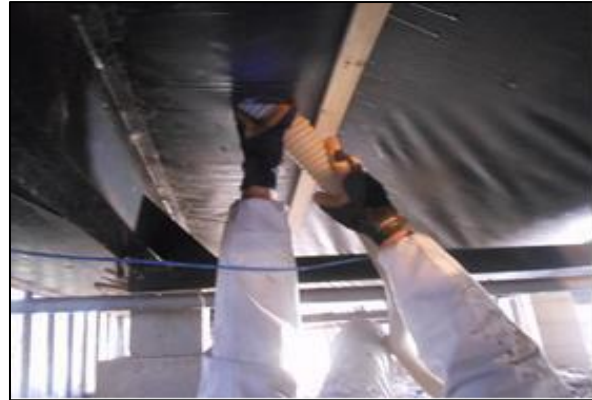
Blowing insulation from under the home: A large diameter fill tube fills cavities rapidly from underneath.
