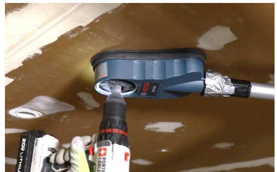
Lead-safe drilling: Using a shrouded drill with a HEPA vacuum removes dust where it is generated.
