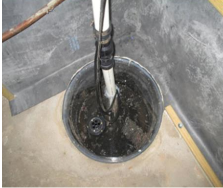
Sump crock – clear cover-sealed
