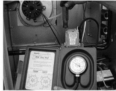
Adjusting gas pressure: Adjusting gas pressure is the only way to change the fuel-air mixture.
