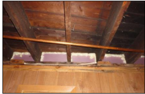
Insulating and air sealing rim joist: Rigid board insulation installed in joist cavities, with spray foam to seal at the edges.
