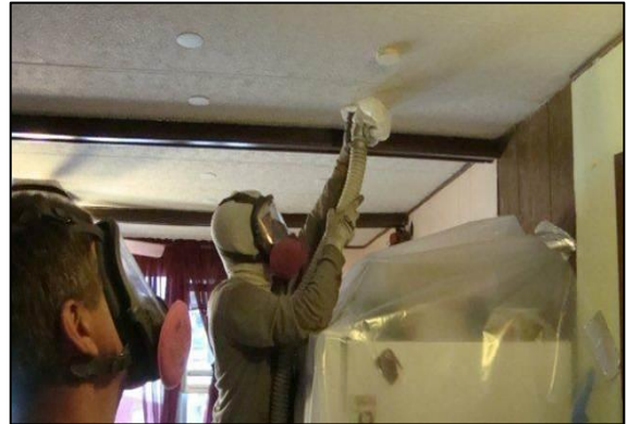
Installing insulation through the ceiling: The technician pushes the fill tube into the cavity and out near the edge of the roof. The holes are drilled in a straight line for aesthetics.
