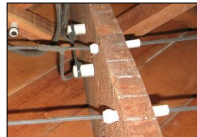
Knob-and-tube wiring: Prior to insulating around knob-and-tube wiring, barriers must be installed to keep insulation at least 3 inches from the wires.
