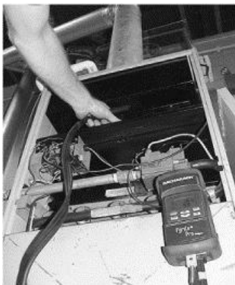
Testing older furnaces: Insert the probe into the draft diverter near the exhaust ports of the heat exchanger.
