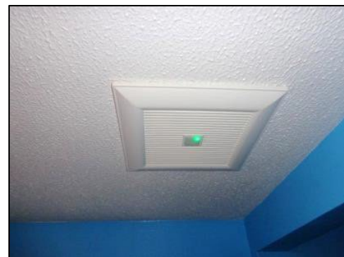
Surface-mounted exhaust fan: Exhaust fans aid air quality by drawing fresh air into the building as they remove indoor pollutants.
