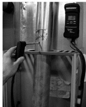
Testing 80+ furnaces: Drill a quarter-inch hole in the metal vent connector to sample combustion gases.
