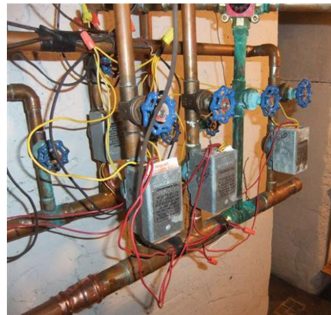
Zone valves: A separate thermostat controls each zone valve. When a thermostat calls for heat, the boiler fires and the zone valve opens.
