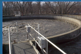
Waste Water Treatment Facilities/Plants (WWTF/P)
